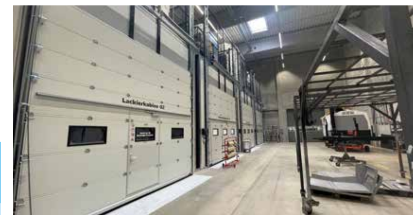
Two preparation and two painting cabins are part of the new paint line. Blasted components are painted in the customer's desired color in four process steps (body painting as standard). Heat recovery is achieved by means of high-efficiency heat wheels.
