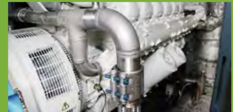
The core of the new system: the cogeneration unit.
