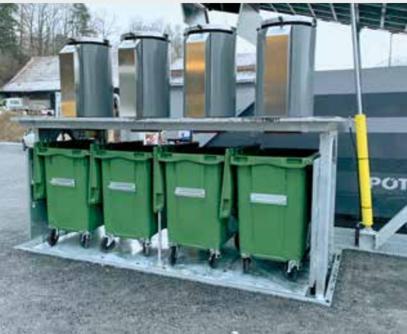
Underground compost/organic waste containers from Contena Ochsner with a Villiger Liftomat system
